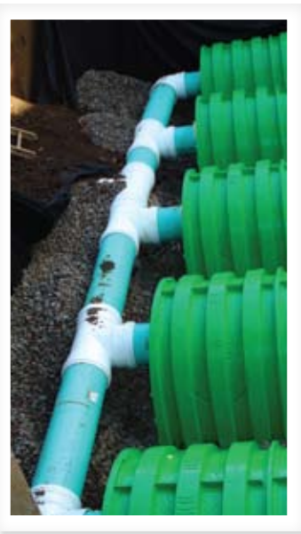
A pipe manifold system was used to distribute stormwater to the chamber rows.
