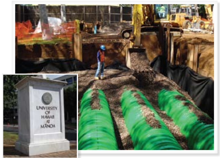
The design flexibility and large storage capacity of the Triton chambers allowed project managers to work within a footprint small and reduce environmental impact on mature trees and landscape during construction.
