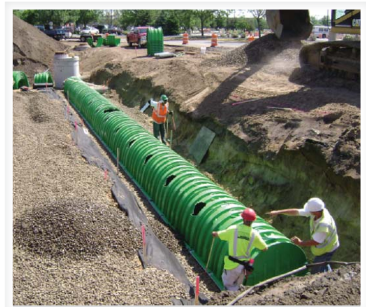
The Triton Main Header Row is assembled on the sediment base in a very confined site. The system's flexible and modular design were key benefits of the installation.
