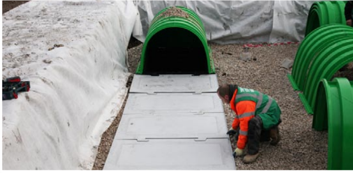
Special sediment floors are placed under the Main Header Row, making maintenance efficient and hassle-free.
