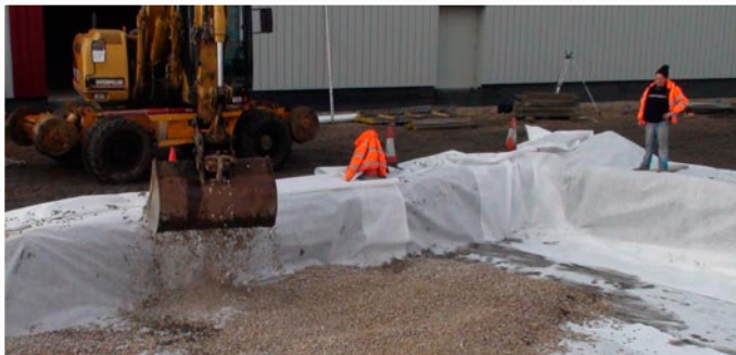
Site preparation with crushed stone and Class II Geofabric was the most time-consuming portion of the whole project.
