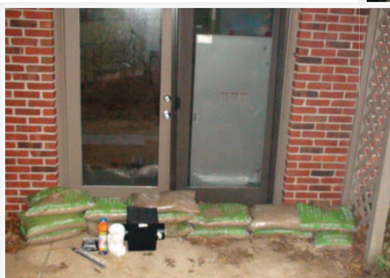
Home owner Brent Zinn resorted to sand bags to try to keep water out of his basement.
