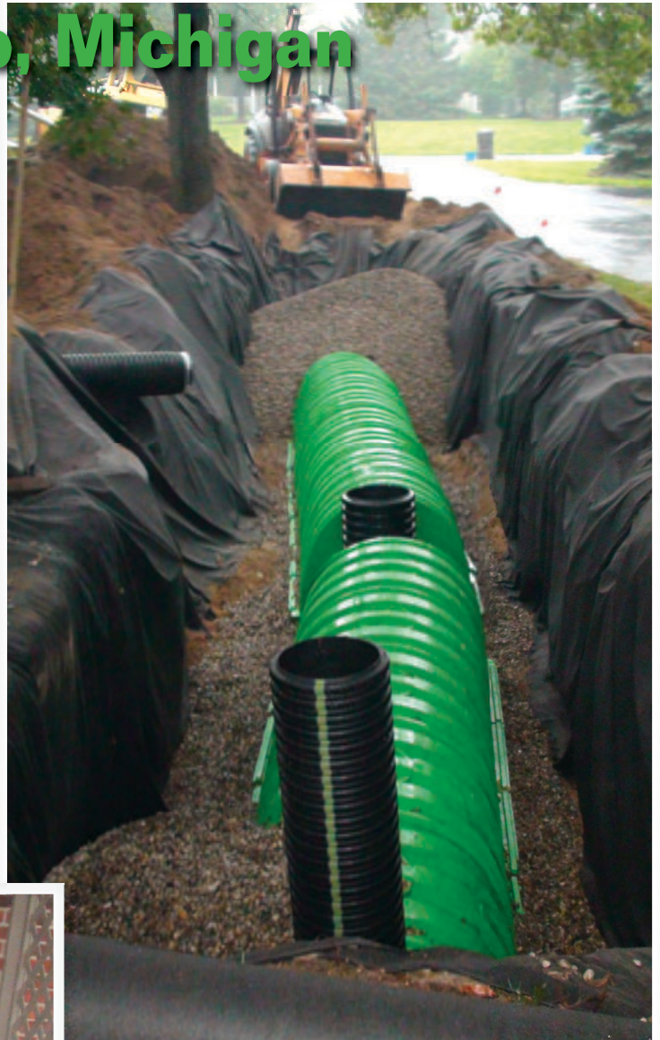
The Triton system will mitigate the stormwater and seasonal water run-off problem. Sixteen chambers, with two sump basins and two dumpsters can hold 6,410 gallons of water.
