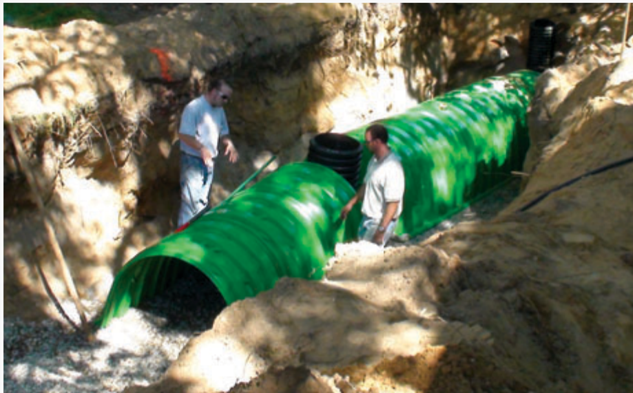
A 45' long x 8' wide trench was dug in tight confines. The four person team completed the installation in three days. Once covered, the Triton water retention system will be completely hidden, providing peace of mind to the homeowner.
