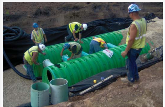
Triton's modular design was the perfect solution to handle the tight space requirement of the road widening project.
