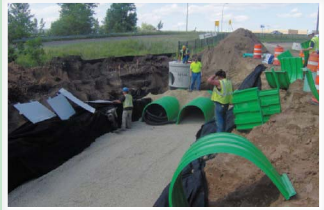
The site required three separate filtration systems for a total volume of 8,500 cubic feet.
